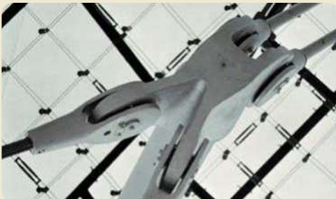
Nodal points of suspended roof construction of the Olympic Stadium in Munich, Germany
